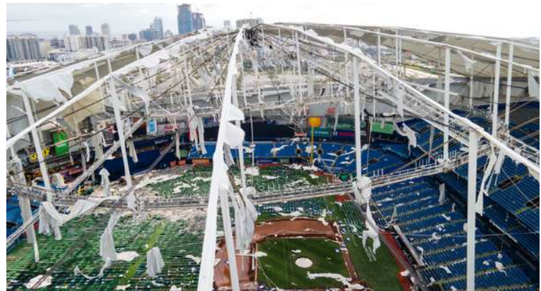
The roof of the Tropicana Field is damaged the morning after Hurricane Milton hit the region, Thursday, Oct. 10, 2024, in St. Petersburg, Fla. (AP Photo/Julio Cortez)
